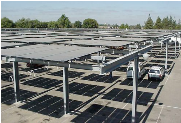
Single-axis sun-tracking solar carport at Cal Expo Fairgrounds in Sacramento, CA
