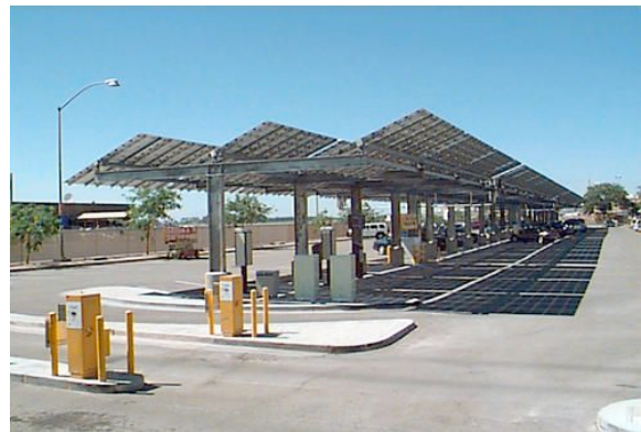
Single-axis sun-tracking solar carport at Sacramento Airport
